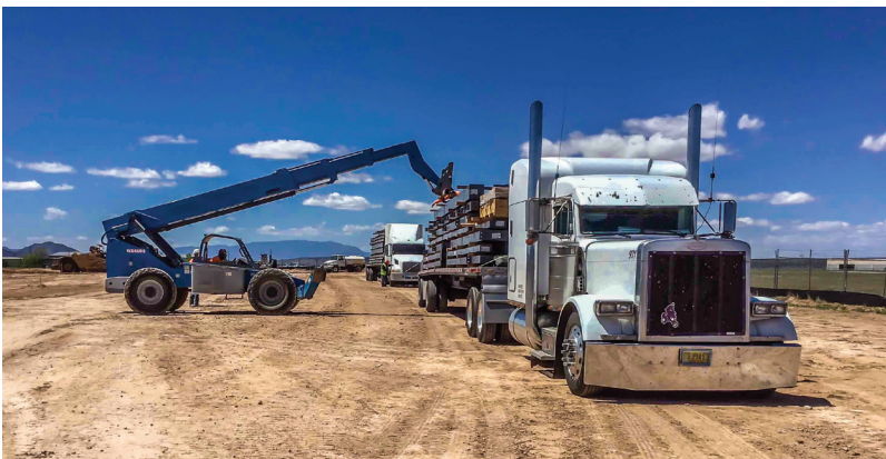
The hangars will be constructed of Butler® pre-engineered steel, totaling 33,000 square feet. The steel recently arrived to the job site on 18 semi trucks!
